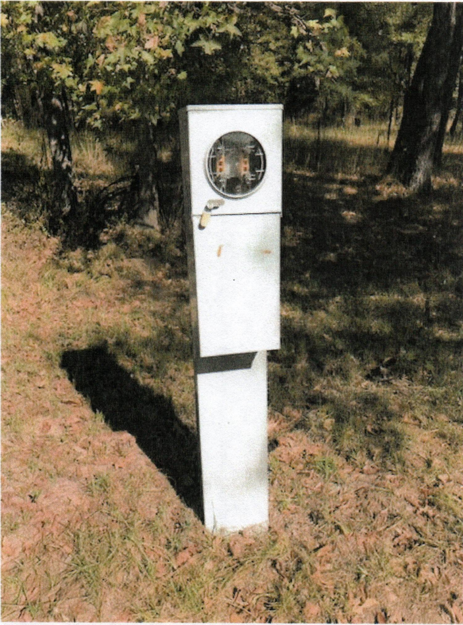
200 Amp Meter Pedestal
